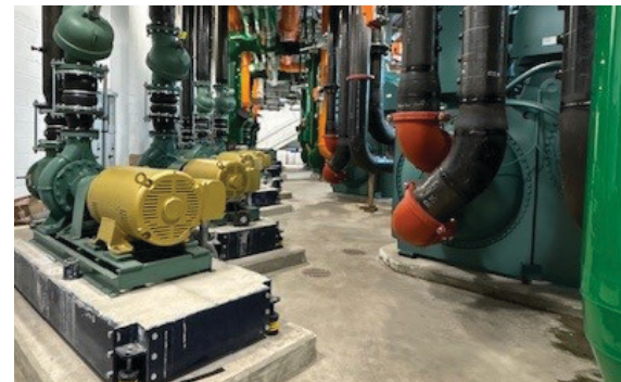
Mechanical Room Finished Installation
